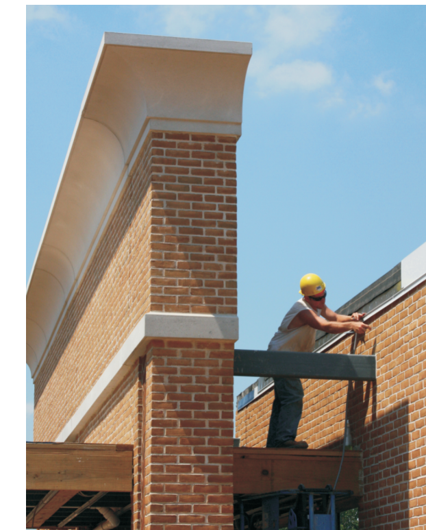
A construction worker puts the finishing touches on the exterior of the Career Programs Building.
